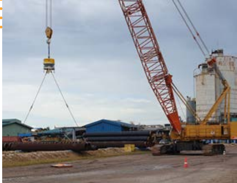
A Roborigger unit lifting pipe by Shawcor in Batam, Indonesia. Photo credit: Roborigger
